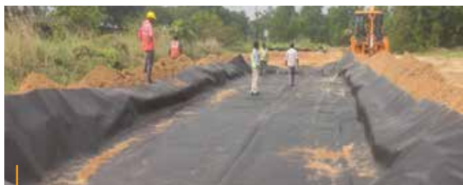
Dug the soil up to 1.5 feet of depth Area: 25 Meters of length and 4 Meters of width The plastic sheet was layered and filled with better soil up to 1 foot level
