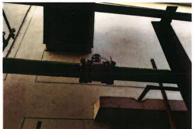
Flow Meter at DFDS
