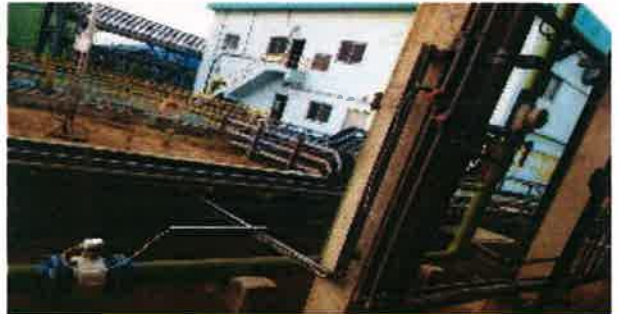
Flow meter at SPDS
