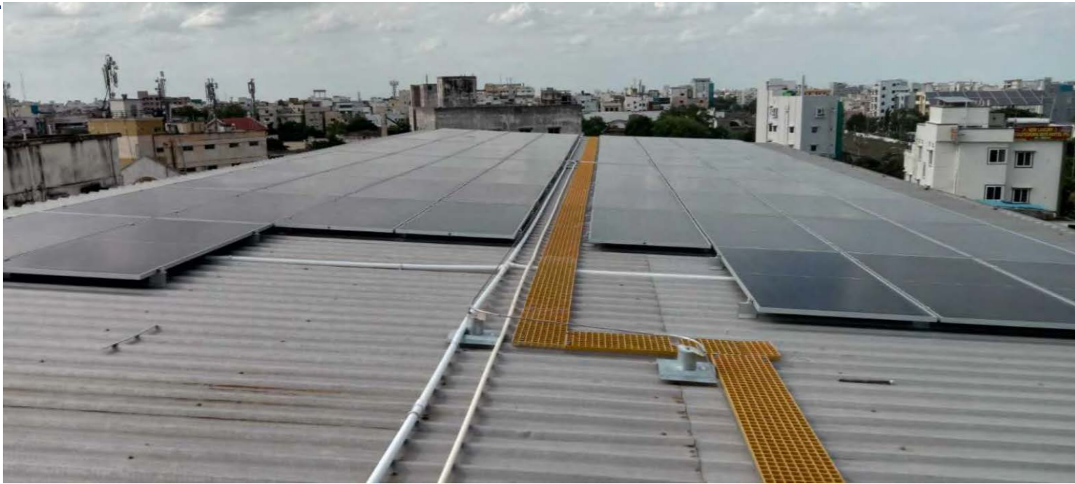
JAYABHARAT HOSPITAL – 50 kWp
