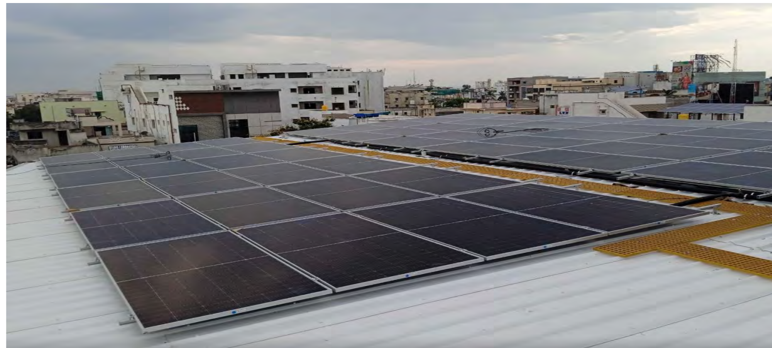
PEOPLES POLYCLINIC -100 kWp
