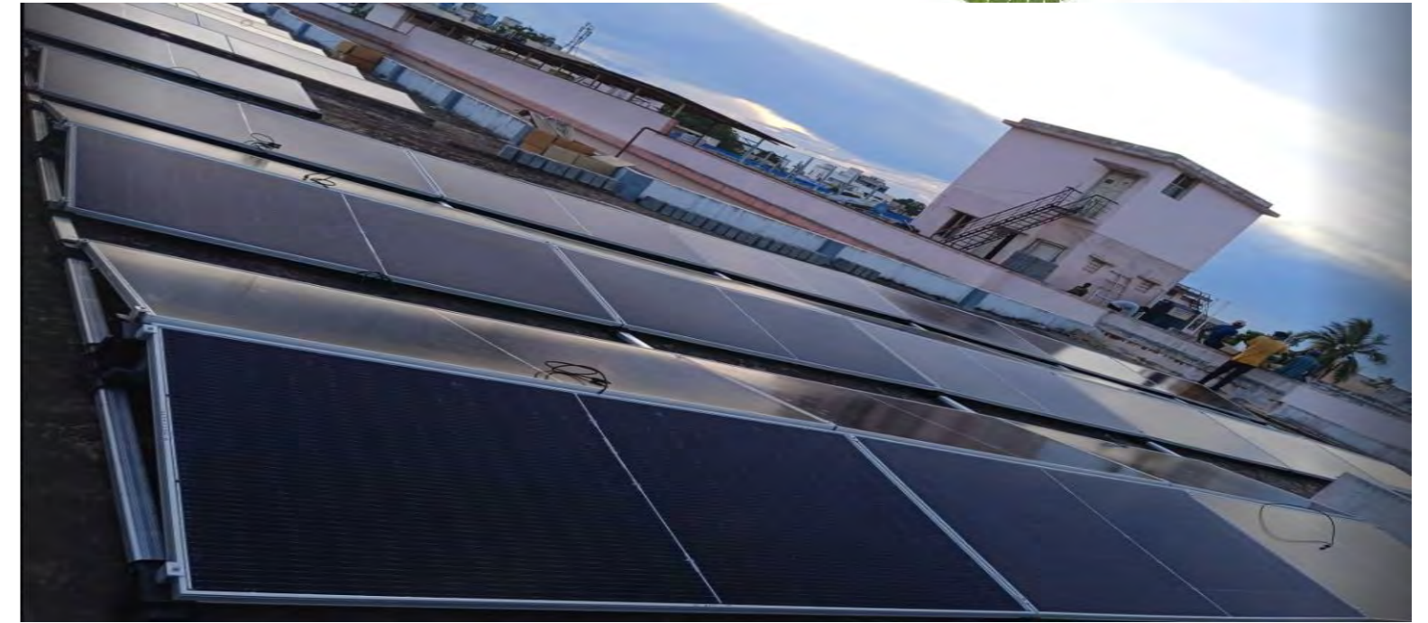
ST JOSEPH HOSPITAL -100 kWp
