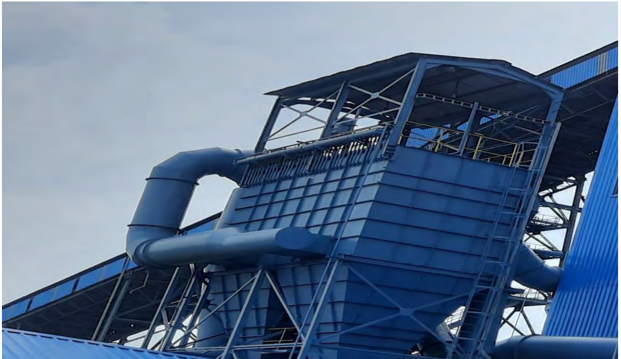
DUST EXTRACTION SYSTEM AT TRANSFER POINTS
