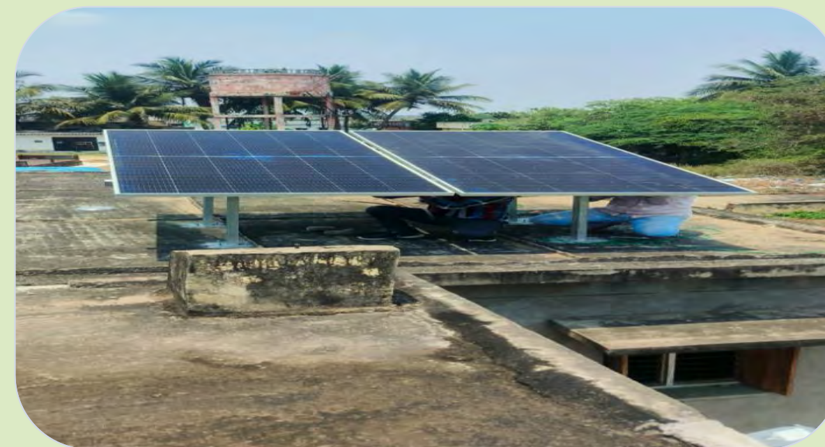
Off-grid solar on Anganwadi center
