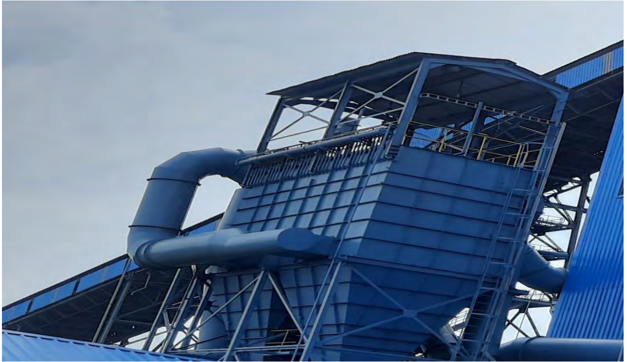
DUST EXTRACTION SYSTEM AT TRANSFER POINTS
