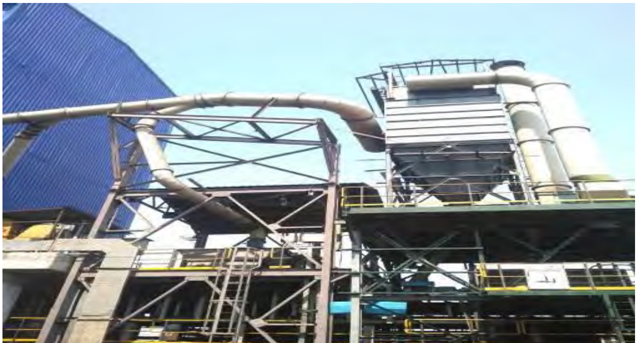
DUST EXTRACTION SYSTEM AT TRANSFER POINTS
