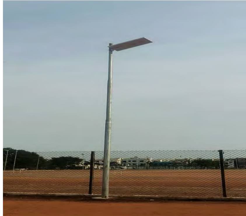
SOLAR STREET LIGHTS AT DISTRICT SPORTS STADIUM
