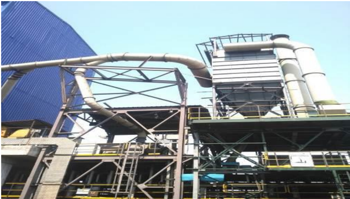
DUST EXTRACTION SYSTEM AT TRANSFER POINTS
