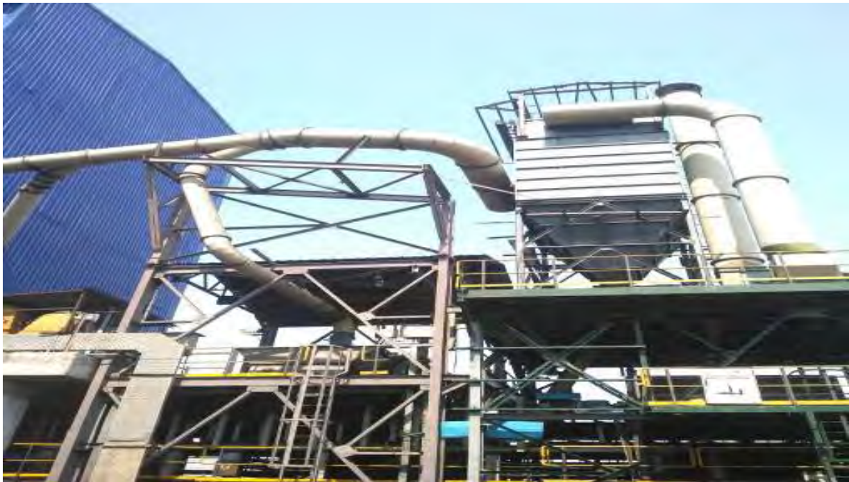
DUST EXTRACTION SYSTEM AT TRANSFER POINTS
