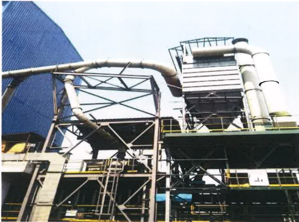
DUST EXTRACTION SYSTEM AT TRANSFER POINTS
