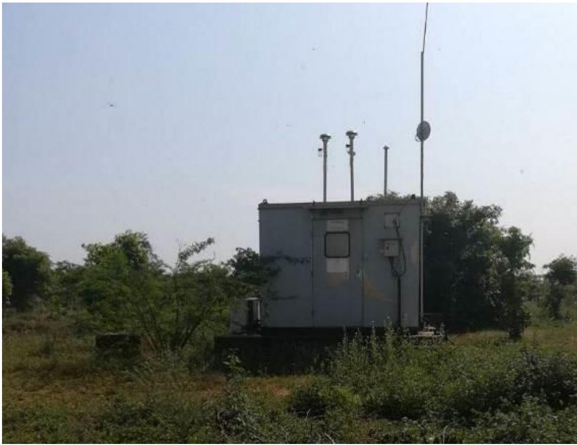
CONTINUOUS AMBIENT AIR QUALITY MONITORING STATION INSIDE THE PLANT
