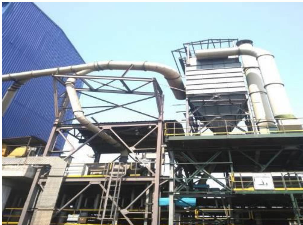
DUST EXTRACTION SYSTEM AT TRANSFER POINTS
