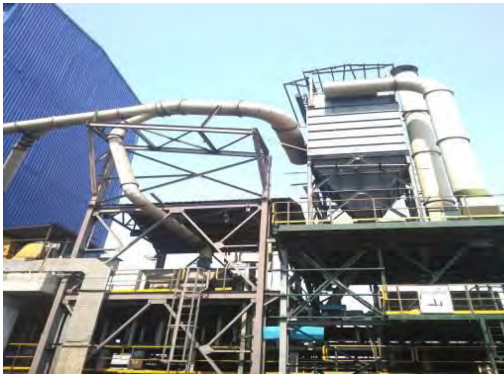
DUST EXTRACTION SYSTEM AT TRANSFER POINTS
