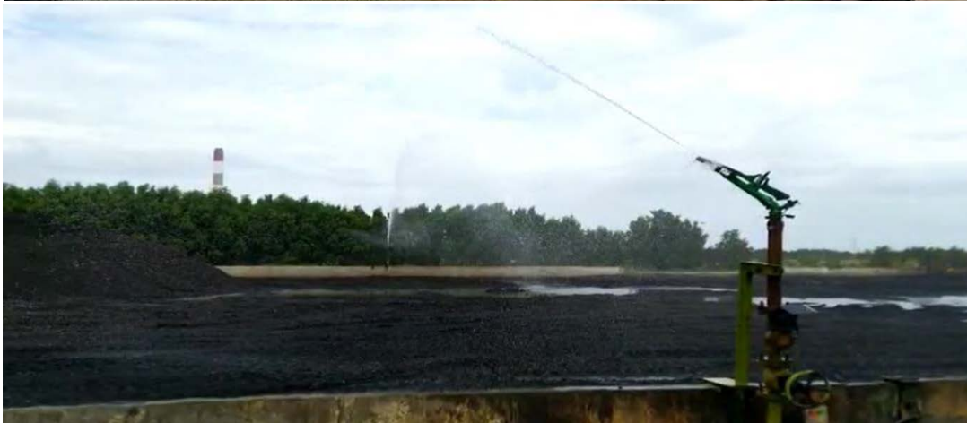
COAL YARD WATER SPRINKLING
