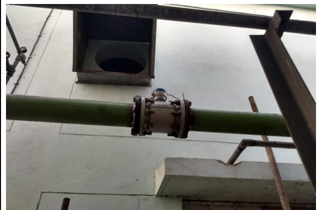
Flow Meter at DFDS
