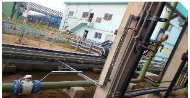
Flow meter at SPDS
