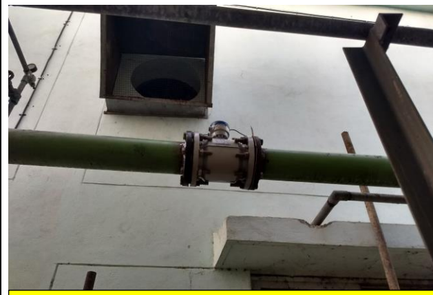
Flow Meter at DFDS
