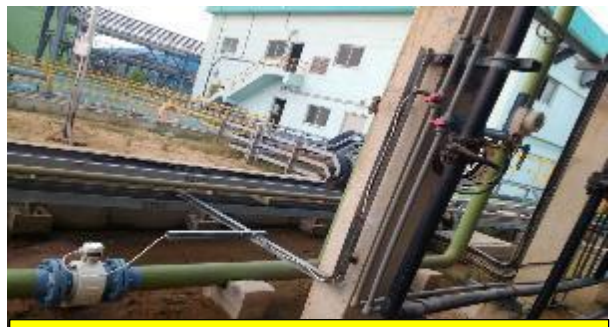
Flow meter at SPDS
